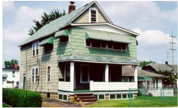
Enclosure of second floor porch has disrupted the structural and visual balance of the structure. The second story looks out of proportion to the first story.
