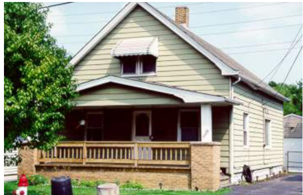
Non-original balustrade looks architecturally inconsistent with the rest of the structure.
